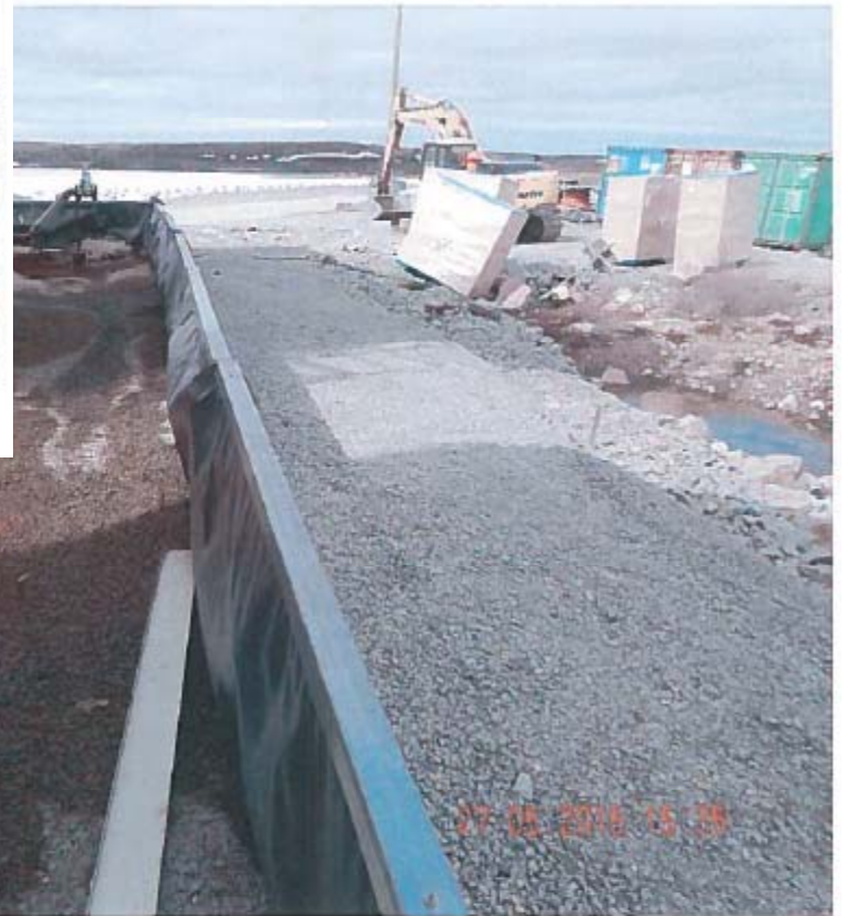
Photo 18 – 500,000L Tank Farm – Area within the main tank farm containment is significantly contaminated with hydrocarbons and requires a clean-up.
