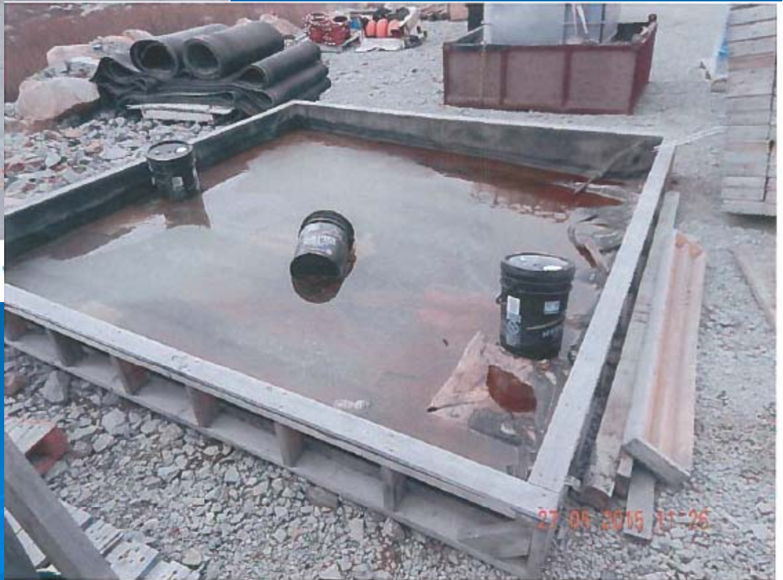
Photo 2 - Water World Building 53 – A containment tray used for hydrocarbon storage was filling with water and will need to be pumped out before it overflows.
