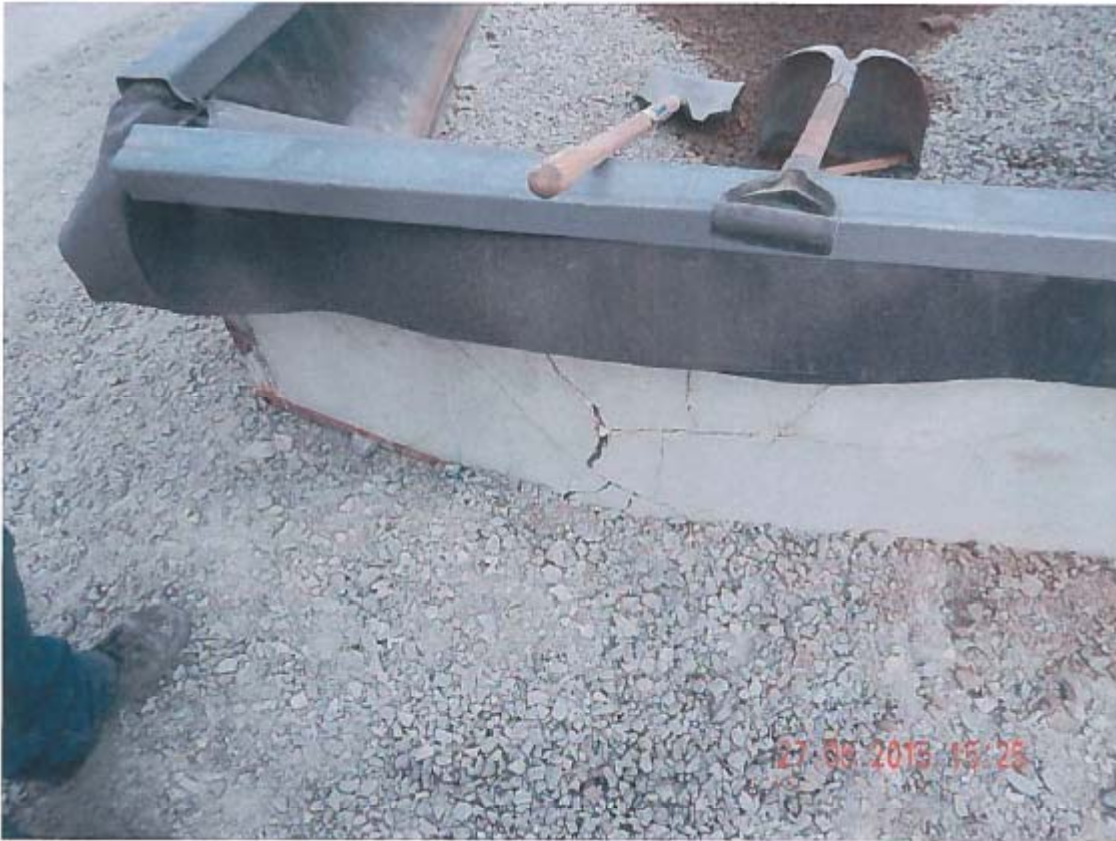
Photo 16 – 500,000L Tank Farm – Containment berm around the fill up module is significantly damaged.
