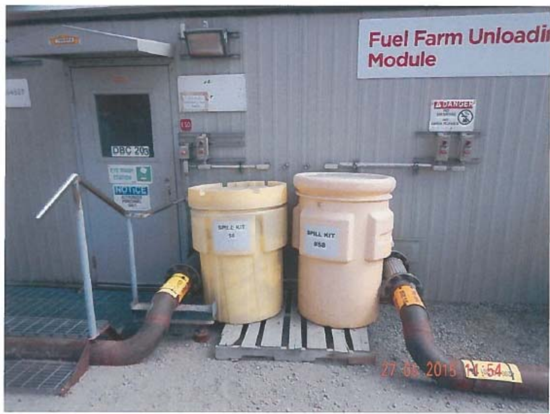
Photo 10 – Fuel Farm Unloading Module Building 31 – Spill kits in place are fully stocked and easily accessible.
