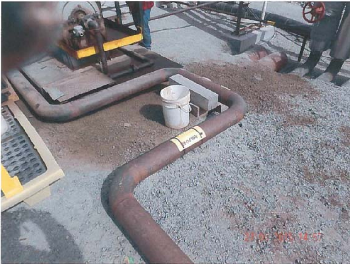
Photo 12 – Fuel Farm Unloading Module Building 31 – Area around the hose reel is heavily stained with hydrocarbons. Clean-up of the area is required.
