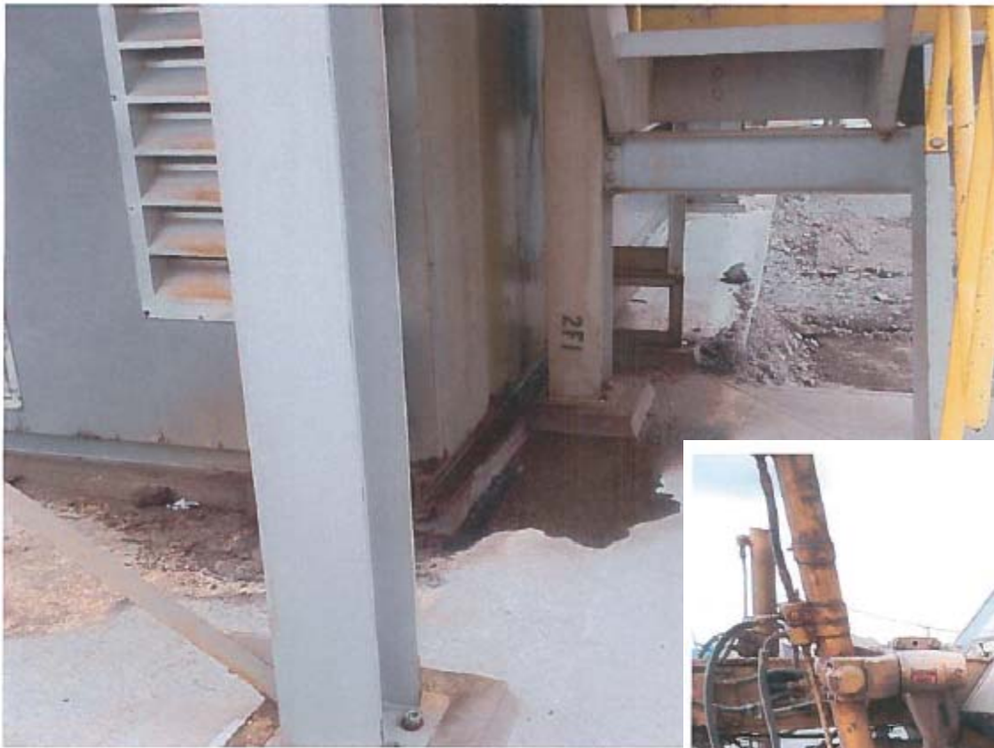
Photo 4 – Fresh Air Raise – Some seepage from the fresh air raise is pooling up outside. The source of the seepage is not known by De Beers at this time. The area is being acted on a regular basis.
