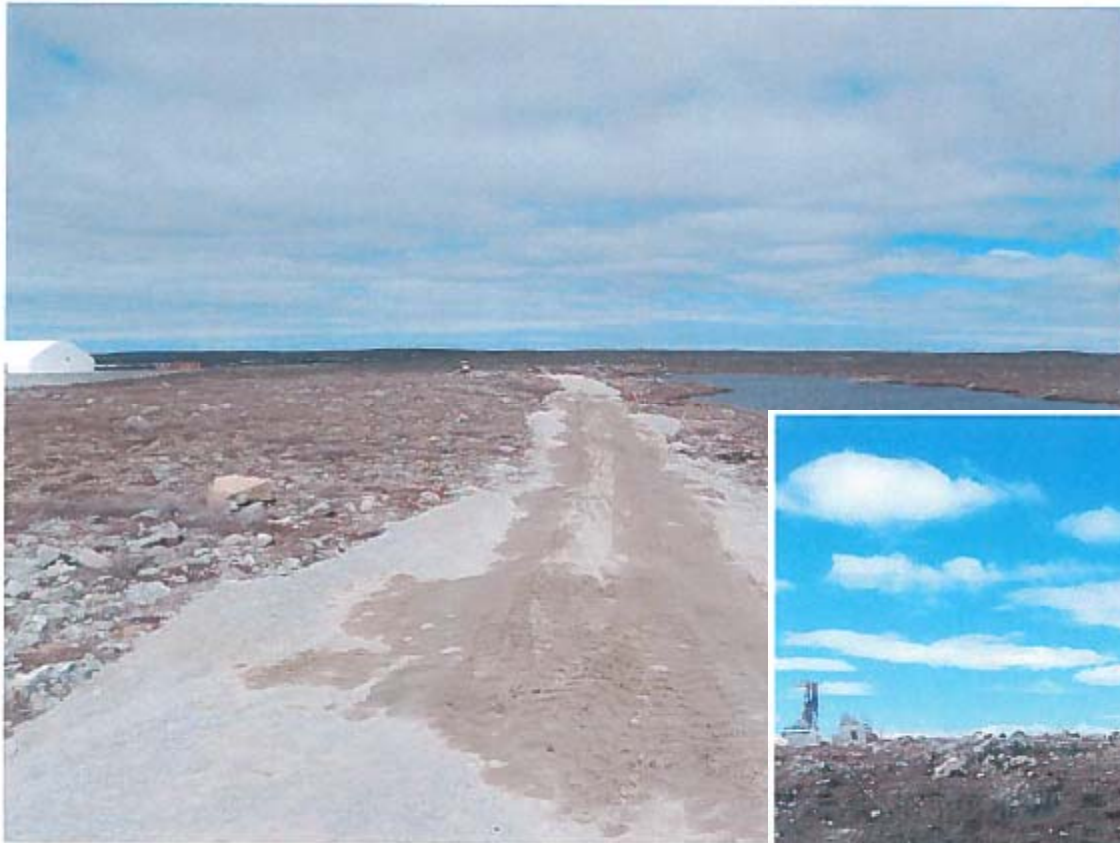
Photo 33 – North Pile West Cell – Perimeter Road for the West Cell is being constructed.
