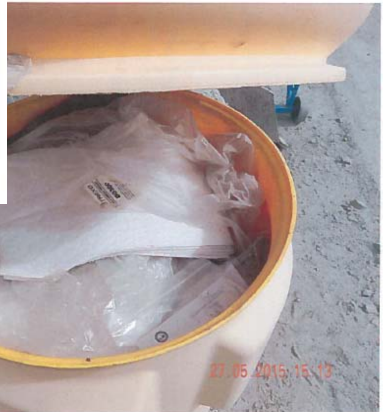
Photo 13 – Fuel Farm LV Module Building 35 – Spill kit fully stocked and easily accessible.
