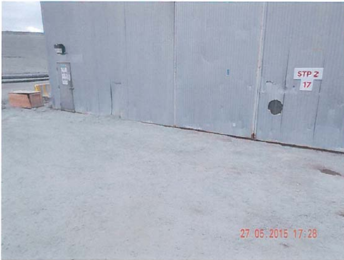
Photo 27 – STP 2 – NT Spill #15-176 - A 30 L sewage spill outside of the Sewage Treatment Plant resulted from a power outage. The spill site has been cleaned up.
